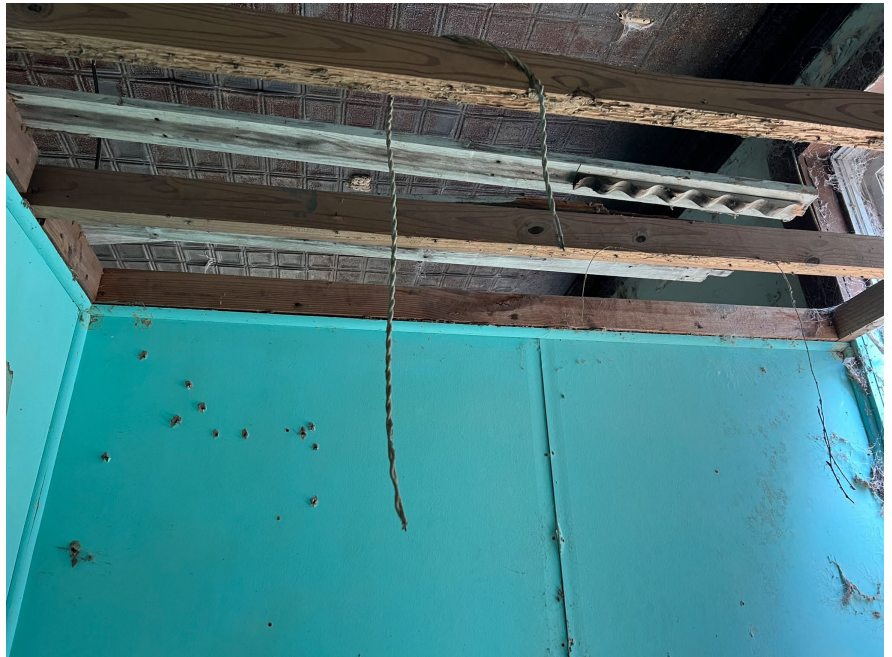
IC.60 Room C - A non-historic ceiling support structure is found in this room
