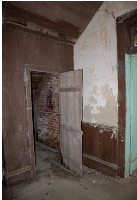
1C.11 Hallway – Door leading into small room under stairs – Minor portion of missing material at the underside of the stairs
