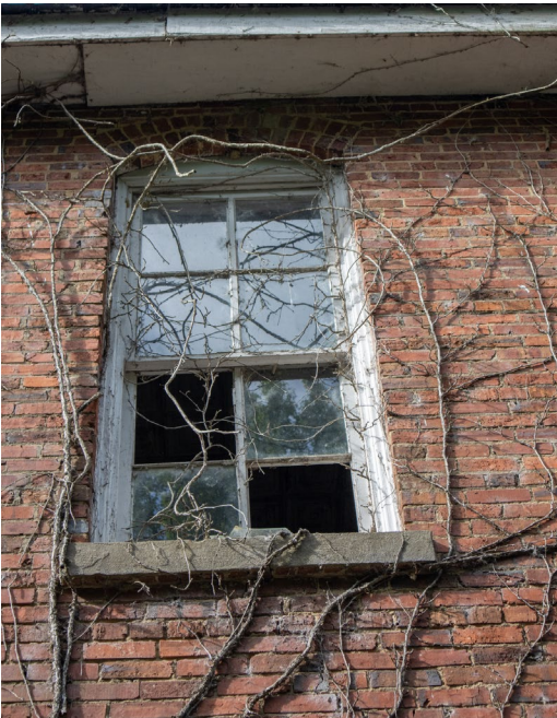
1B.18 North façade – The intrusion of climbing foliage along this side of the building is further weakening the masonry and soffit boards
