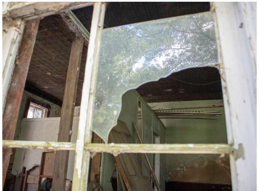
1B.15 West façade – Many windows on this façade contain either cracked or missing lites
