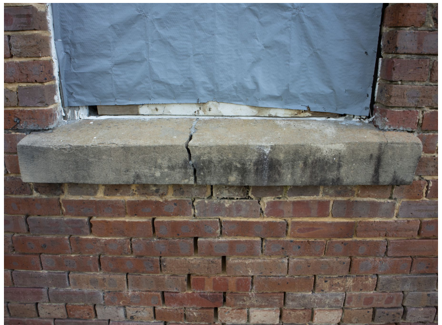
1B.7 South facade - Fracturing of concrete sill casing
