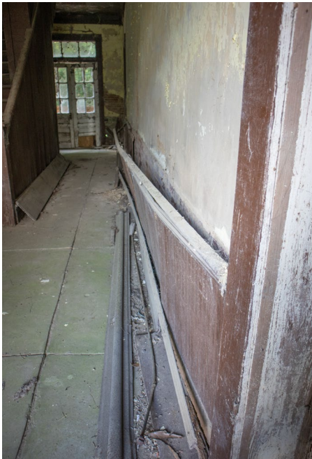
1C.4 Hallway - Beadboard wainscoting falling away from wall exposing masonry below
