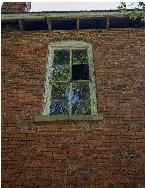
1B.14 West facade – Large portion of missing soffit
