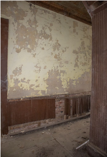
1C.7 Hallway – Beadboard wainscoting falling away from wall exposing masonry below
