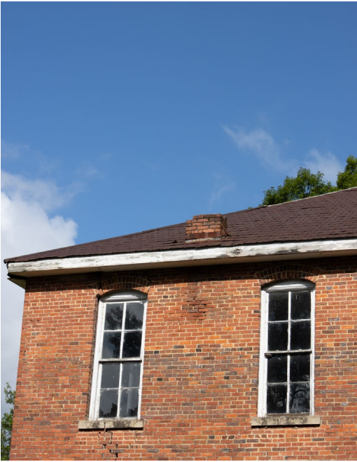
1B.20 East façade – The chimneys on this side of the building are experiencing masonry loss that is disturbing the roofing
