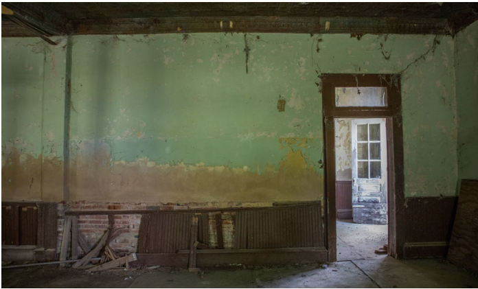
IC.35 Room B – Looking East – Beadboard wainscoting falling away from wall exposing masonry below
