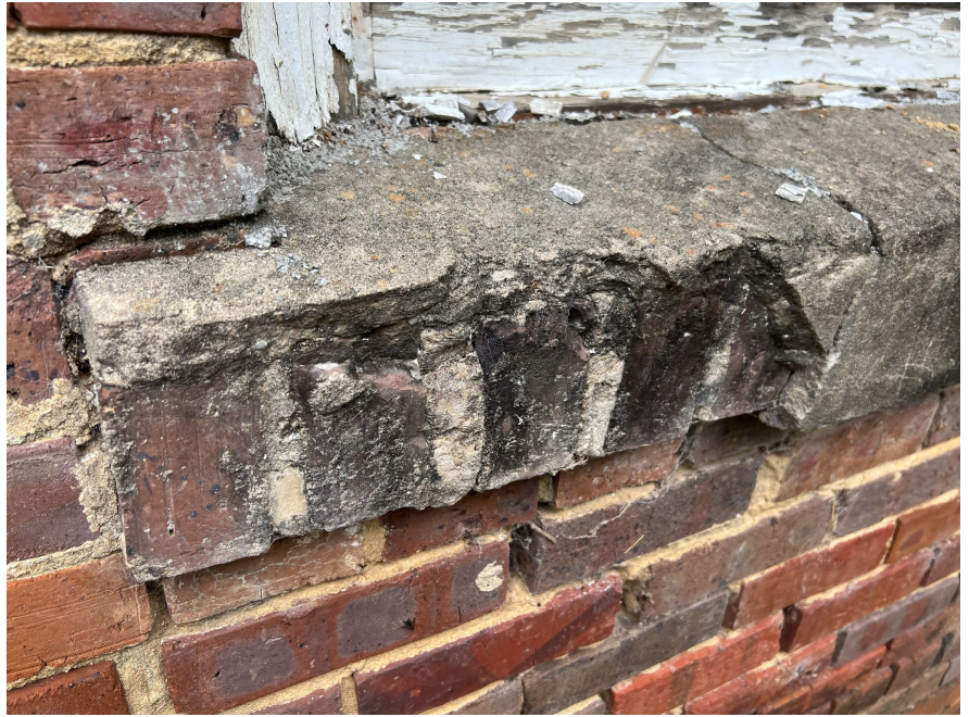
1B.25 East façade – Detail of lower story window concrete sill casing that has major deterioration
