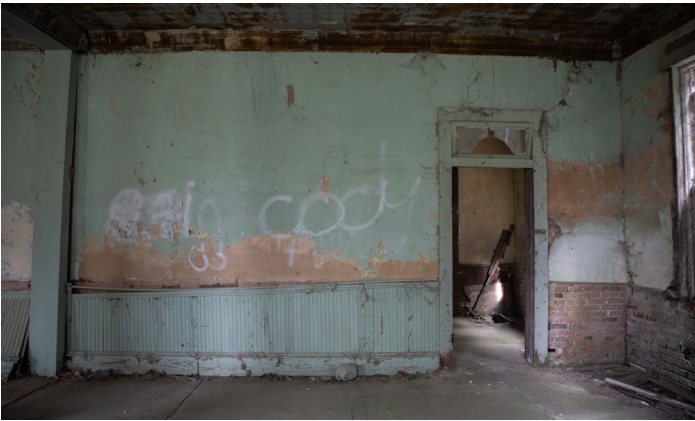
IC.25 Room A – Looking West into hallway - Beadboard wainscoting falling away from wall exposing masonry below
