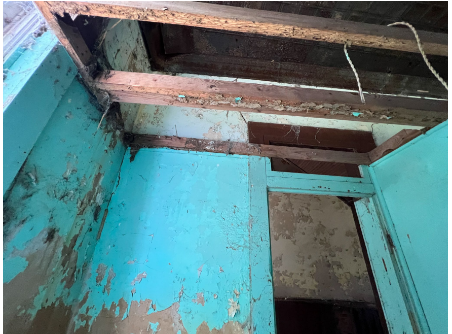
IC.58 Room C - A non-historic ceiling support structure is found in this room
