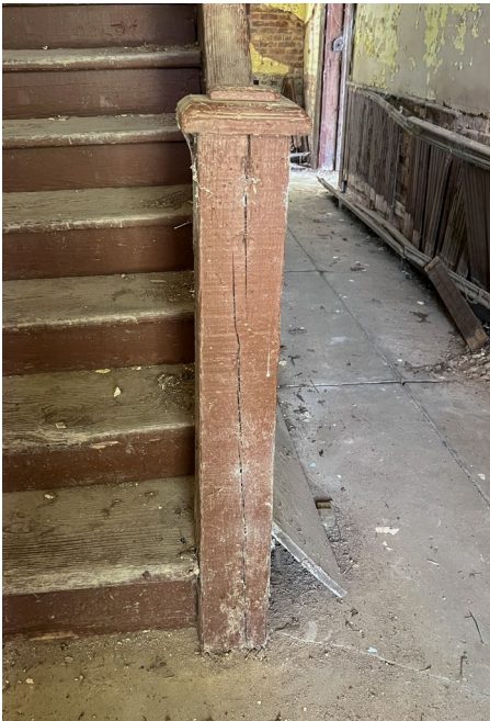
1C.16 Hallway – Newel post is experiencing minor cracking
