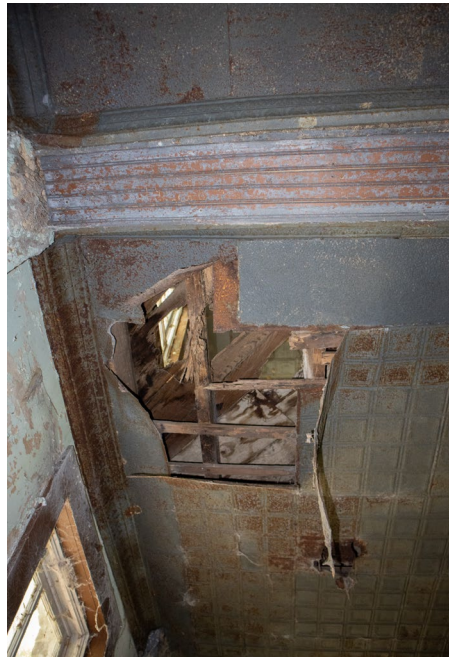
IC.49 Room B – Severe damage in the pressed metal ceiling
