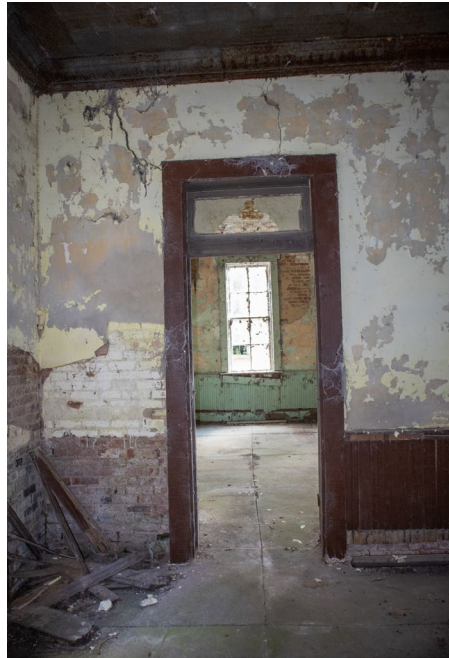
1C.8 Hallway – Opening looking into Room A – Door no longer remains
