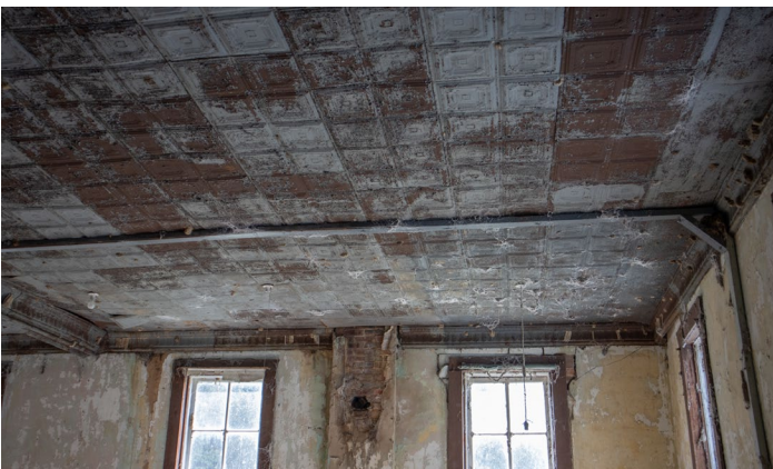
1D.10 Room A – Detail of pressed metal ceiling – The design of the upper story ceiling is just slightly more elaborate than that of the one used on the lower story
