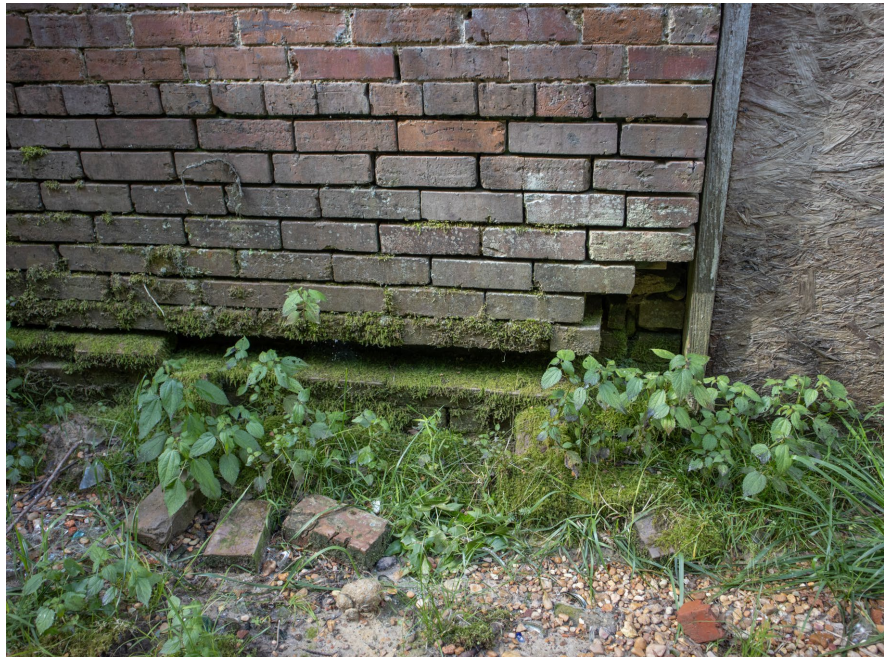
1B.19 North façade – Significant loss of masonry can be found on both sides of rear entrance
