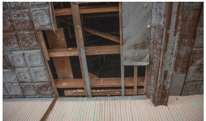
1D.11 Room A – Opening in the upper story ceiling exposing the attic
