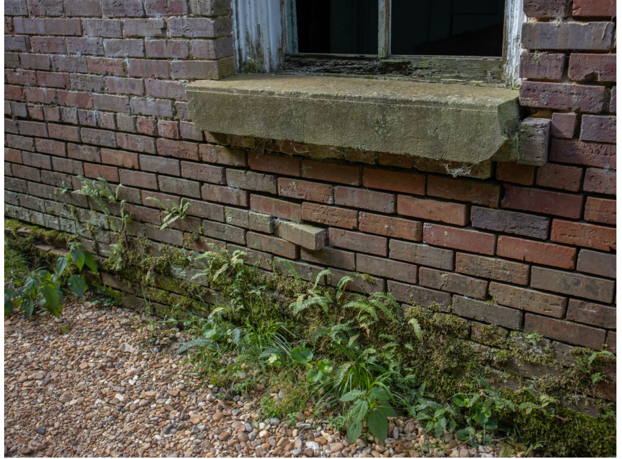
1B.17 North façade – Heavy presence of intrusive lichens, mosses, and other foliage along the bottom portions of building is likely due to improper drainage of rainwater
