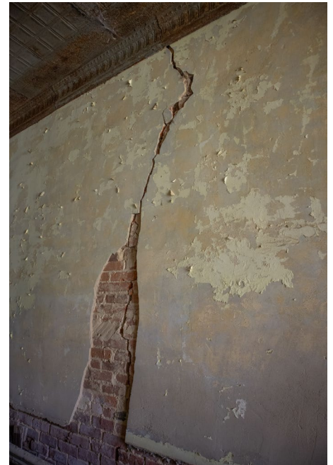
1C.6 Hallway - Detail of plaster delamination exposing cracking masonry below
