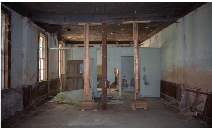
IC.39 Room B – Looking North – The sagging of the main structural beam can best be seen in this image
