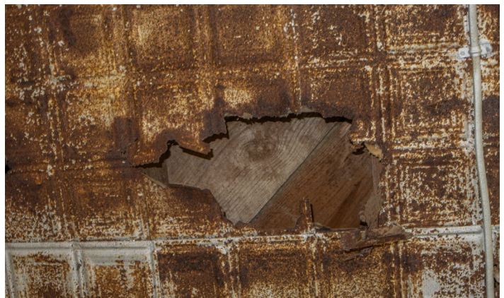
IC.30 Room A – Missing portion of pressed metal ceiling exposing ceiling structure
