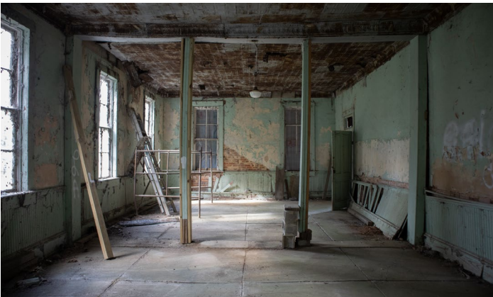
IC.27 Room A – Looking South – Supporting columns have been reinforced – Why would the bottom portion be unpainted on the leftmost one? Are they even original?
