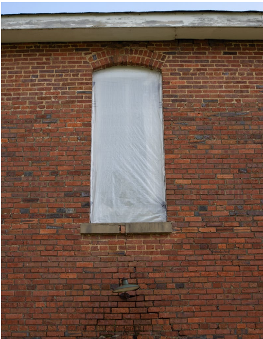
1B.4 South facade – All windows on this facade have been sheathed in plastic as to protect them
