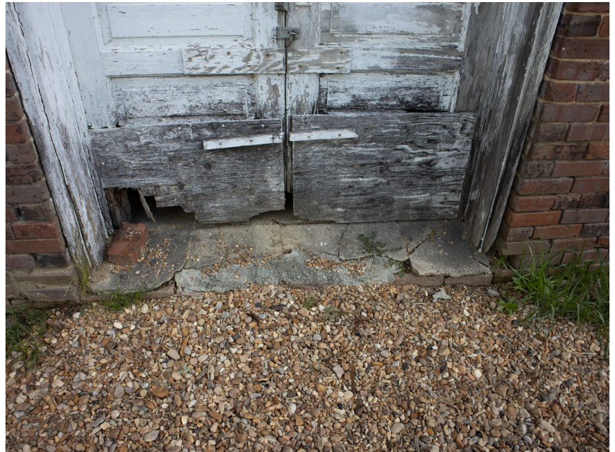
1B.3 South facade entrance door – Severe deterioration of lower portions of the door and concrete threshold
