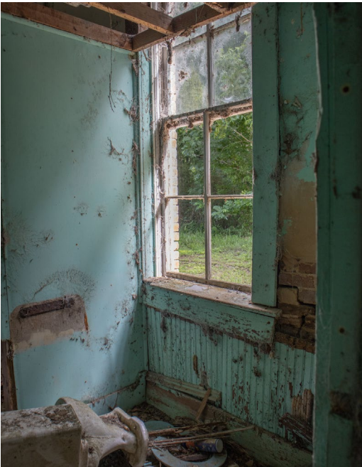
IC.59 Room C - A non-historic ceiling support structure is found in this room
