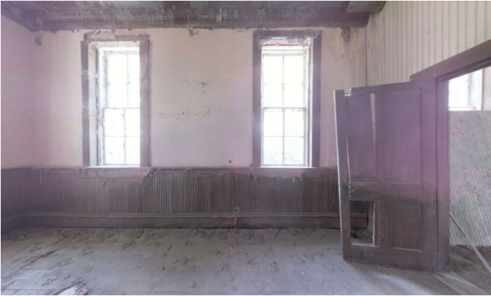
1D.22 Room C – Looking North - Small hole in tongue and groove floor behind door
