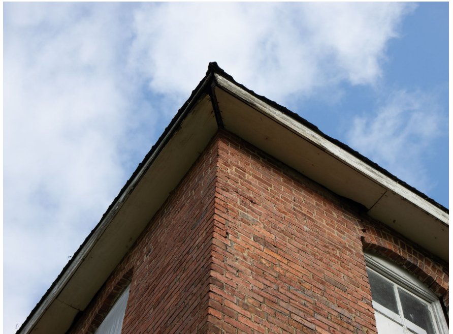
1B.23 East façade – Both the Northeast and Southeast corners of the building are experiencing separation between the soffit and fascia boards due to deterioration of the wood
