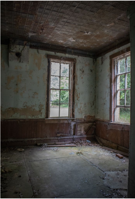
IC.45 Room B - Notice chimney connection
