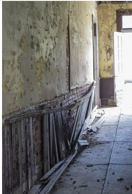
1C.5 Hallway - Beadboard wainscoting falling away from wall exposing masonry below
