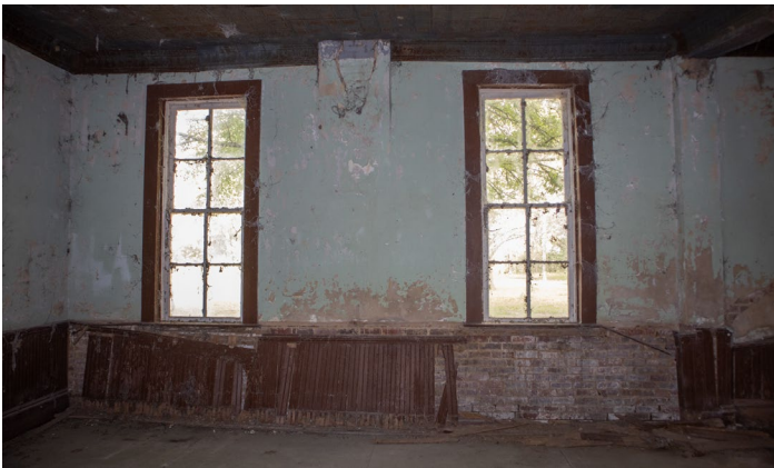
IC.37 Room B – Looking West - Beadboard wainscoting falling away from wall exposing masonry below - Notice chimney connection
