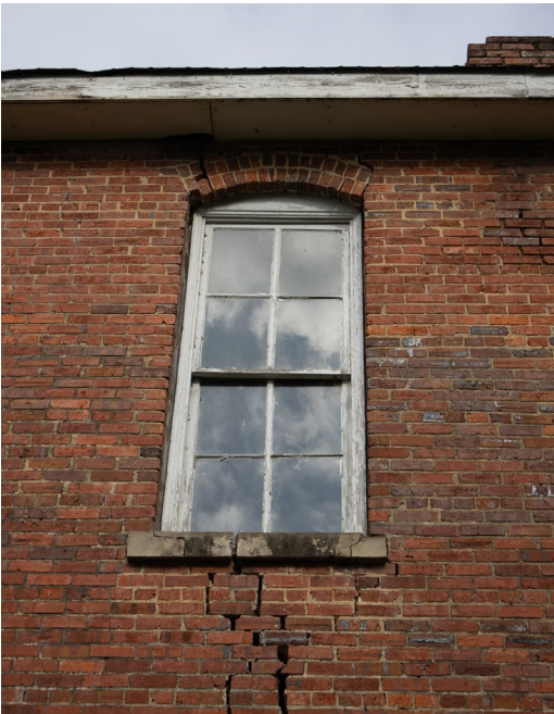
1B.22 East façade – Upper story window is experiencing major separation of masonry above curved lintel and below concrete sill casing
