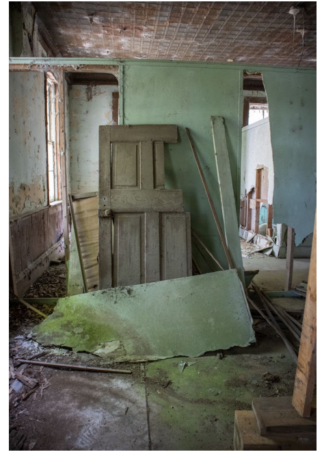
IC.47 Room B – Looking North – What appears to be an original door can be seen in a damaged state
