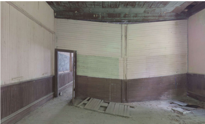
1D.24 Room C – Looking South – Large hole can be found in Southwest corner – There is significant bowing of the partition wall between this room and Room B
