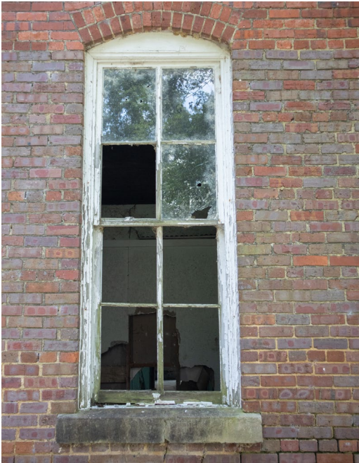
1B.8 West façade – Lower story window experiencing separation between bottom sash rail and its fracturing sill
