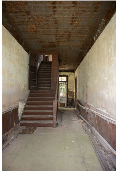
1C.14 Hallway – Looking North toward the rear entrance – Notice missing portion of concrete floor at base of the stairs
