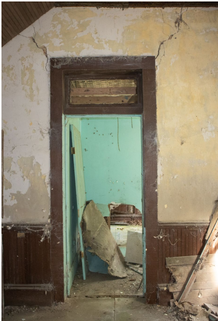
1C.10 Hallway – Opening looking into Room C – Door has been removed from frame
