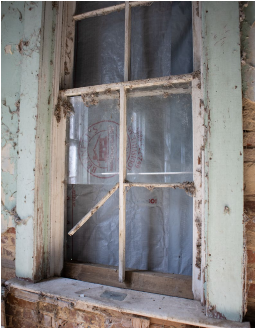
IC.31 Room A – Example of window deterioration
