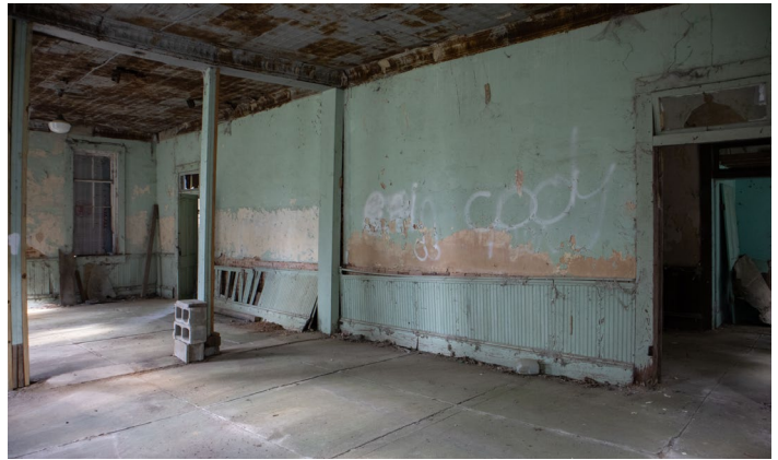
IC.26 Room A – Looking Southwest – Pilaster is separating from masonry wall
