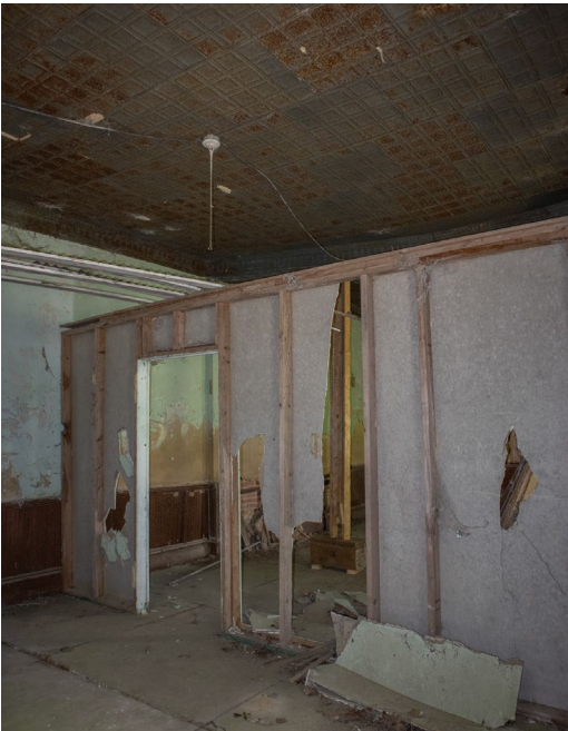
IC.43 Room B – The non-historic half wall partition is made of 2x4 boards and drywall
