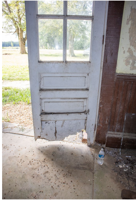
1C.2 Hallway - Severe deterioration of bottom rail and panels on primary entrance doors
