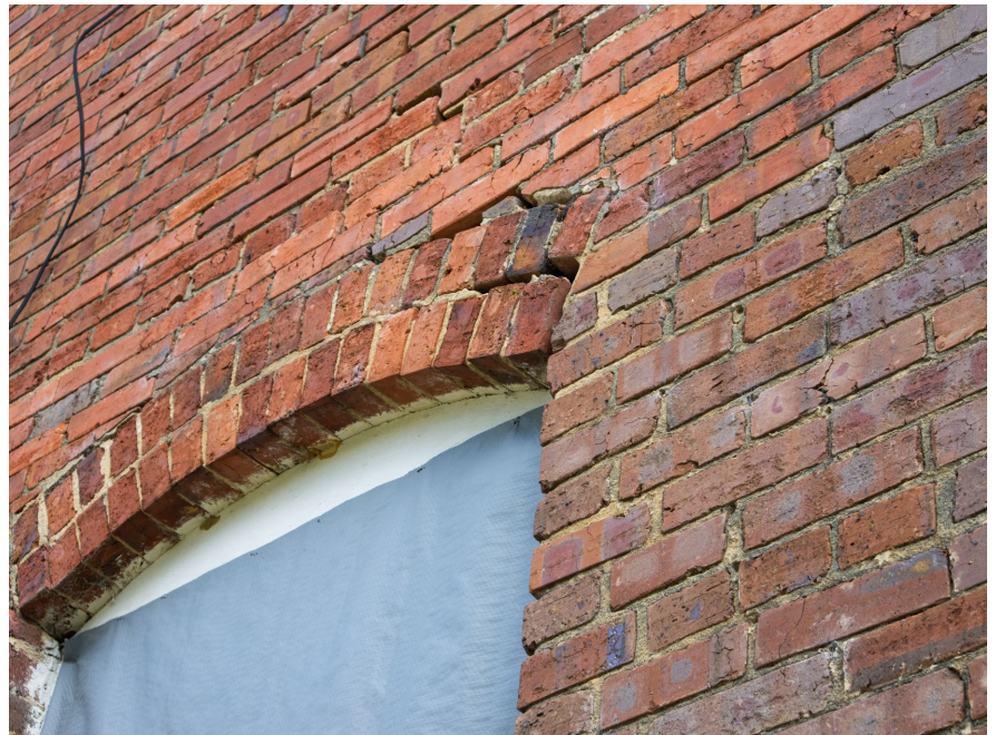
1B.5 South facade – Many locations along this facade are experiencing separation of masonry due to loss of mortar along the window's curved lintels
