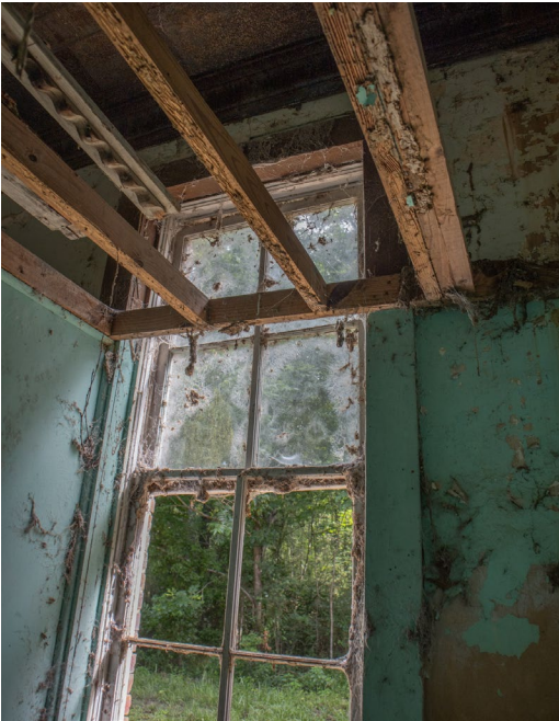
IC.57 Room C – A non-historic ceiling support structure is found in this room
