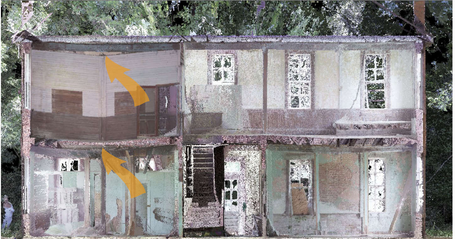
1D.23 Scanned section image – Notice the severe sag in the ceilings and floors on the Western portion of the building
