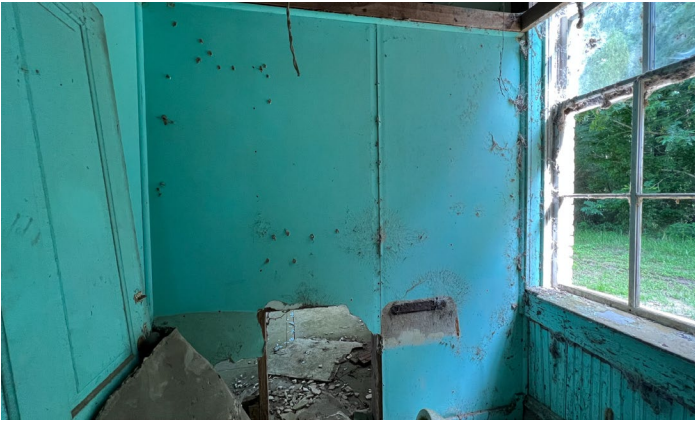
IC.53 Room C – Looking West – The northern and eastern facing walls are made of dywall
