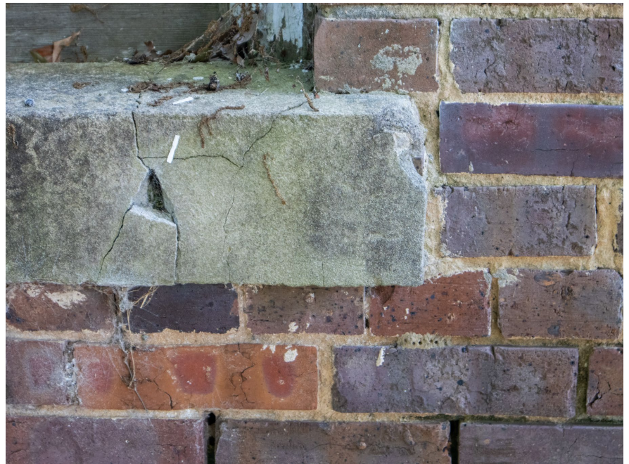
1B.13 West façade – Detail of fracturing concrete sill casing
