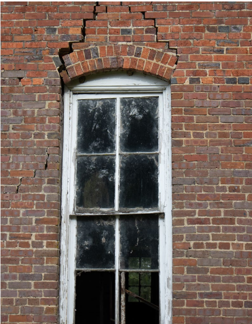
1B.26 East façade – Lower story window that is experiencing major separation between masonry along it's curved lintel
