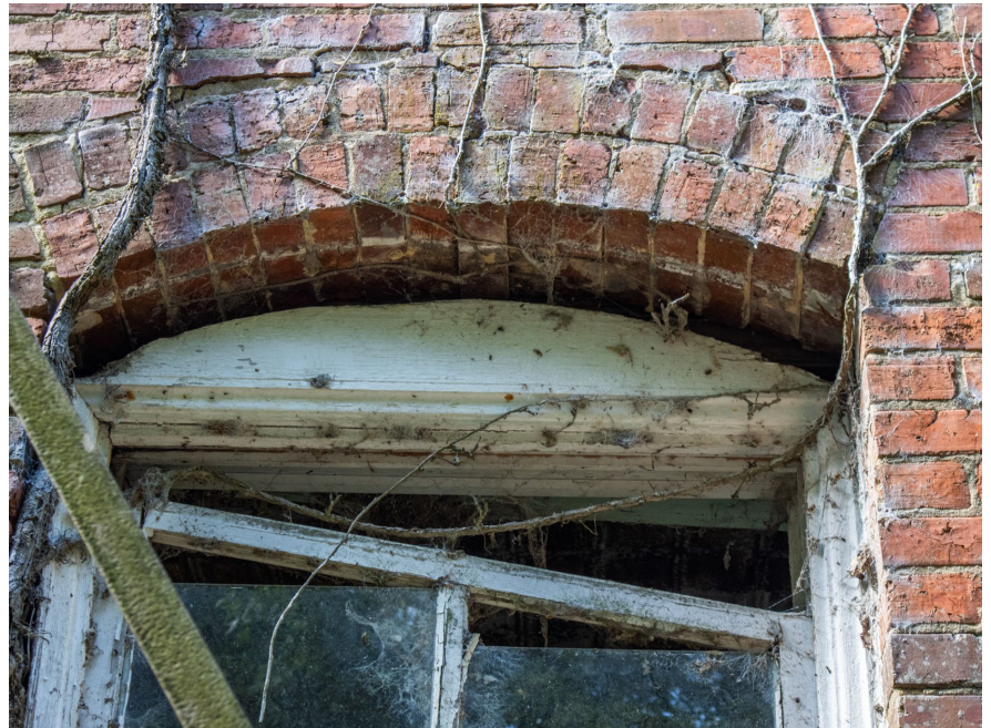
1B.19 North façade – Lower story window experiencing separation between curved lintel and header
