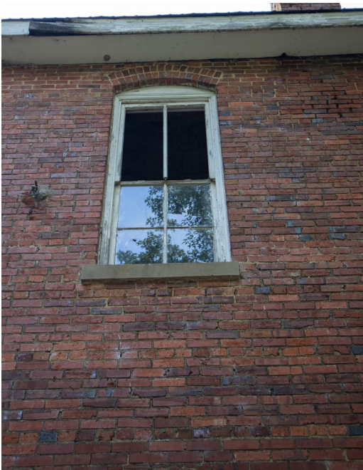
1B.12 West façade – Portions of the fascia boards appear to have water related damage further threatening the attic space
