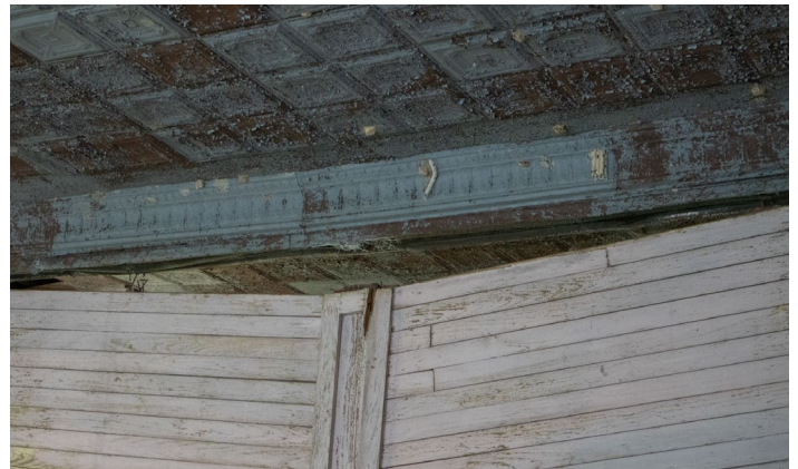
1D.19 Room B – There is significant bowing of the partition wall between this room and Room C
