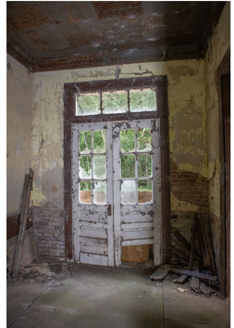
1C.9 Hallway – Rear entrance doors are experiencing deterioration of bottom rail and panels
