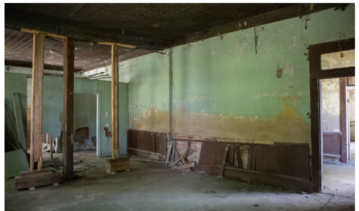
IC.40 Room B - Beadboard wainscoting falling away from wall exposing masonry below - Loss of paint at this level could indicate the former presence of a chalkboard?
