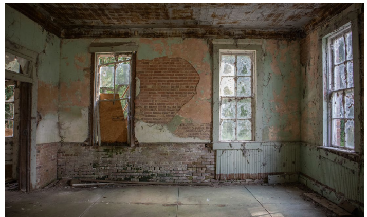
IC.24 Room A – Looking North – Large Portion of Beadboard wainscoting has been removed
