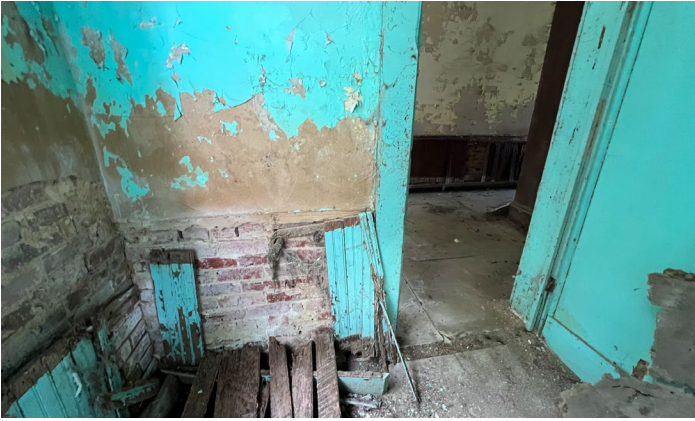
IC.51 Room C – Looking East - Beadboard wainscoting falling away from wall exposing masonry below
