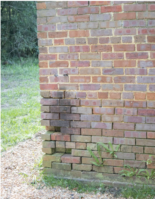
1B.10 Northwest corner – Significant loss of masonry – discoloration of bricks indicates ???
