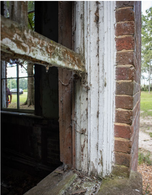
1B.18 North façade – Detail of northwest window deterioration
