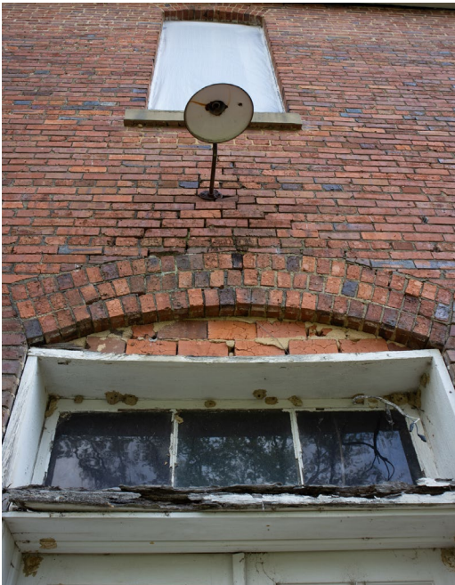
1B.3 South facade entrance door – severe deterioration of header and head jamb causing bowing
