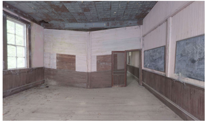
1D.17 Room B – Looking North into Room C – Tongue-and-groove wall is suffering from severe bowing
