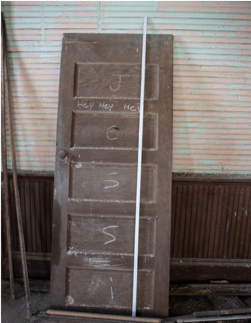
1D.12 Room A – Detail of historic five paneled door that is different in appearance than other doors found in the building
