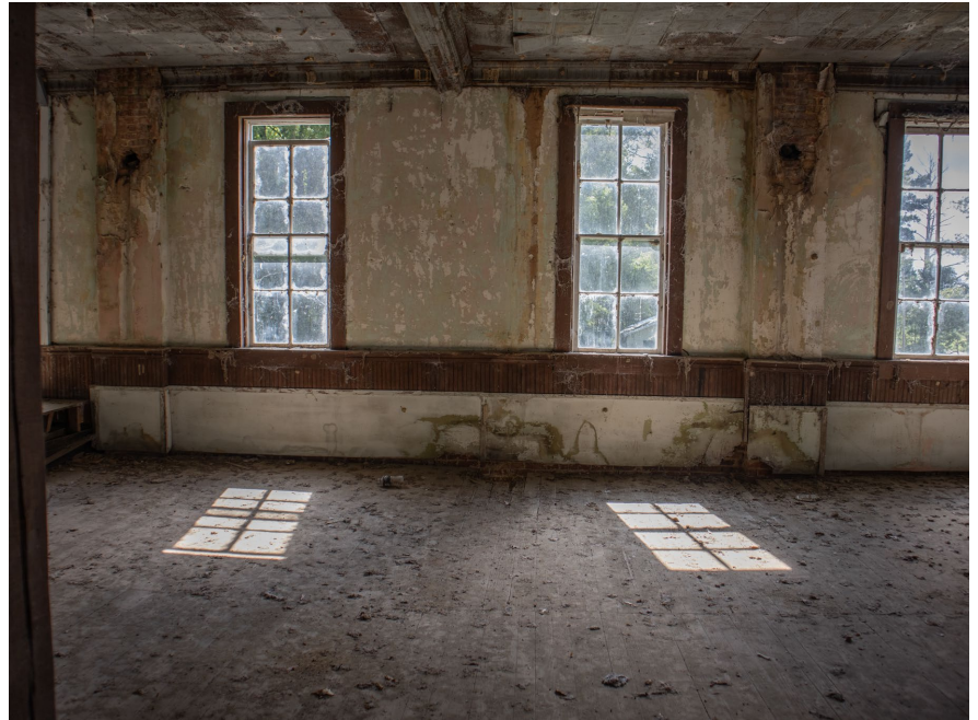
1D.13 Room A – Looking East – Notice chimney connection and water damaged wainscoting
