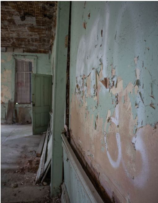
IC.33 Room A - Pilaster column is separating from masonry wall
