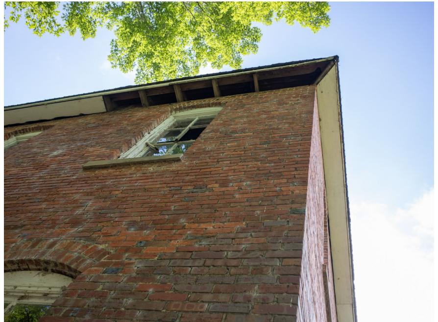
1B.11 Southwest corner – Large portion of missing soffit
