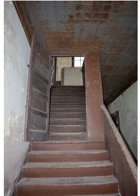
1C.15 Hallway – Detail of walls and door found mid way up the stairs
