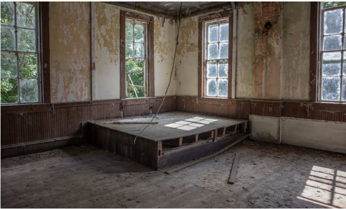
1D.7 Room A – Detail of stage platform – Notice anchors for exterior fire stair
