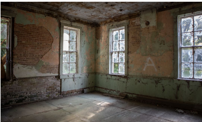
IC.23 Room A – Looking Northeast – Notice chimney connection
