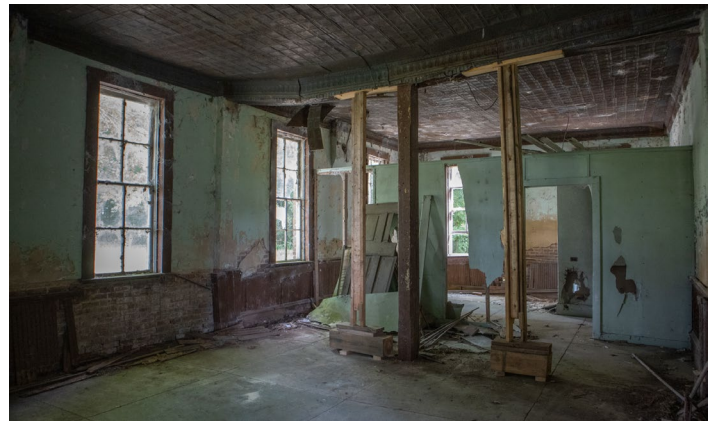
IC.38 Room B – Looking Northwest - Supporting columns have been reinforced using 2x4 boards – center column is unique compared to others
