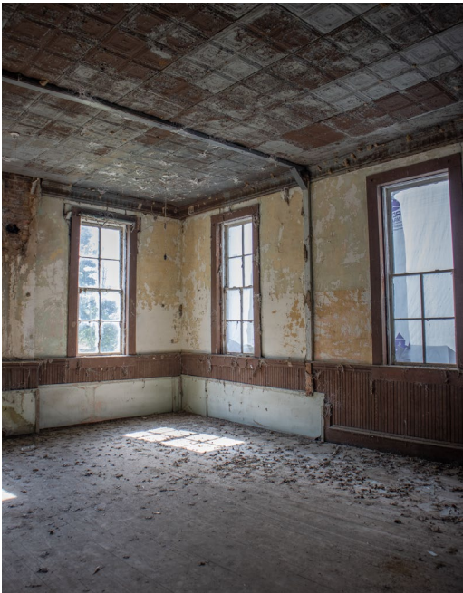
1D.14 Room A – Looking Southeast – A nonoriginal wooden strip masks electrical wires
