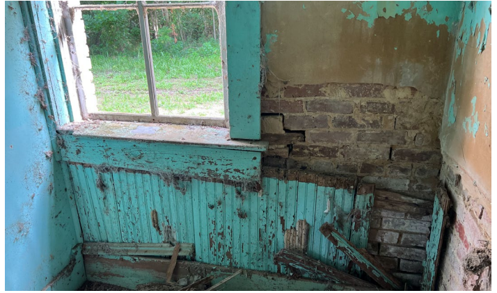
IC.52 Room C – Looking North - Beadboard wainscoting falling away from wall exposing masonry below
