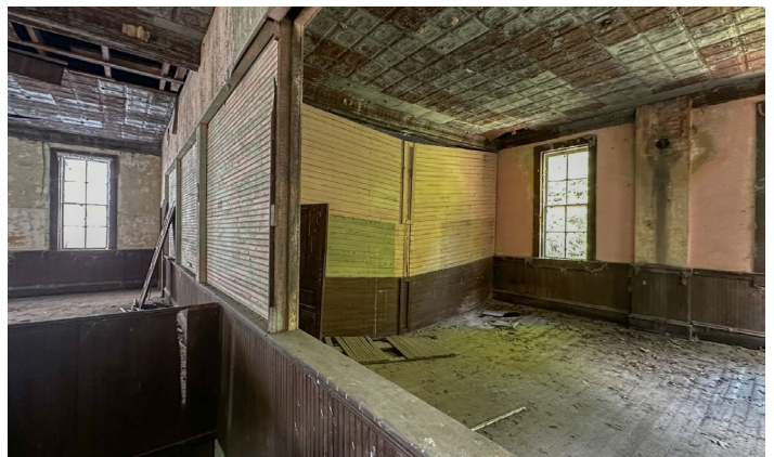
1D.27 Room C – Looking into Room C from top of stairs – Door in this room varies
