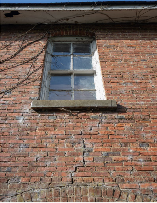
1B.16 North façade – Separation of masonry above rear entrance – Notice protrusion in soffit board
