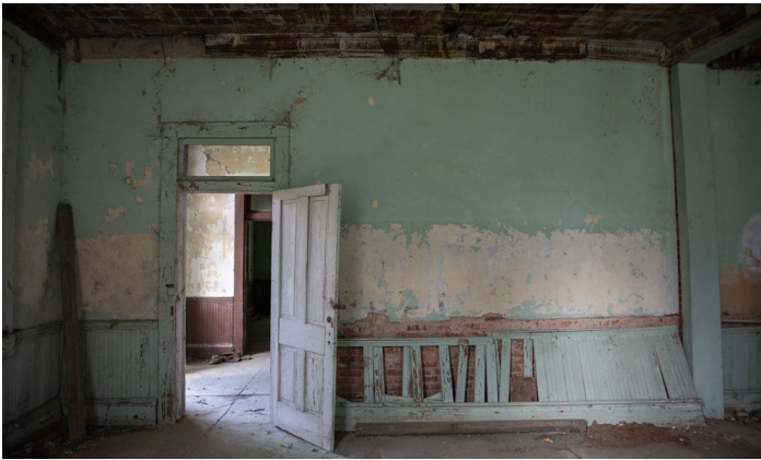
IC.19 Room A – Looking West into the hallway – Beadboard wainscoting falling away from wall exposing masonry below – Loss of paint at this level could indicate the former presence of a chalkboard?
