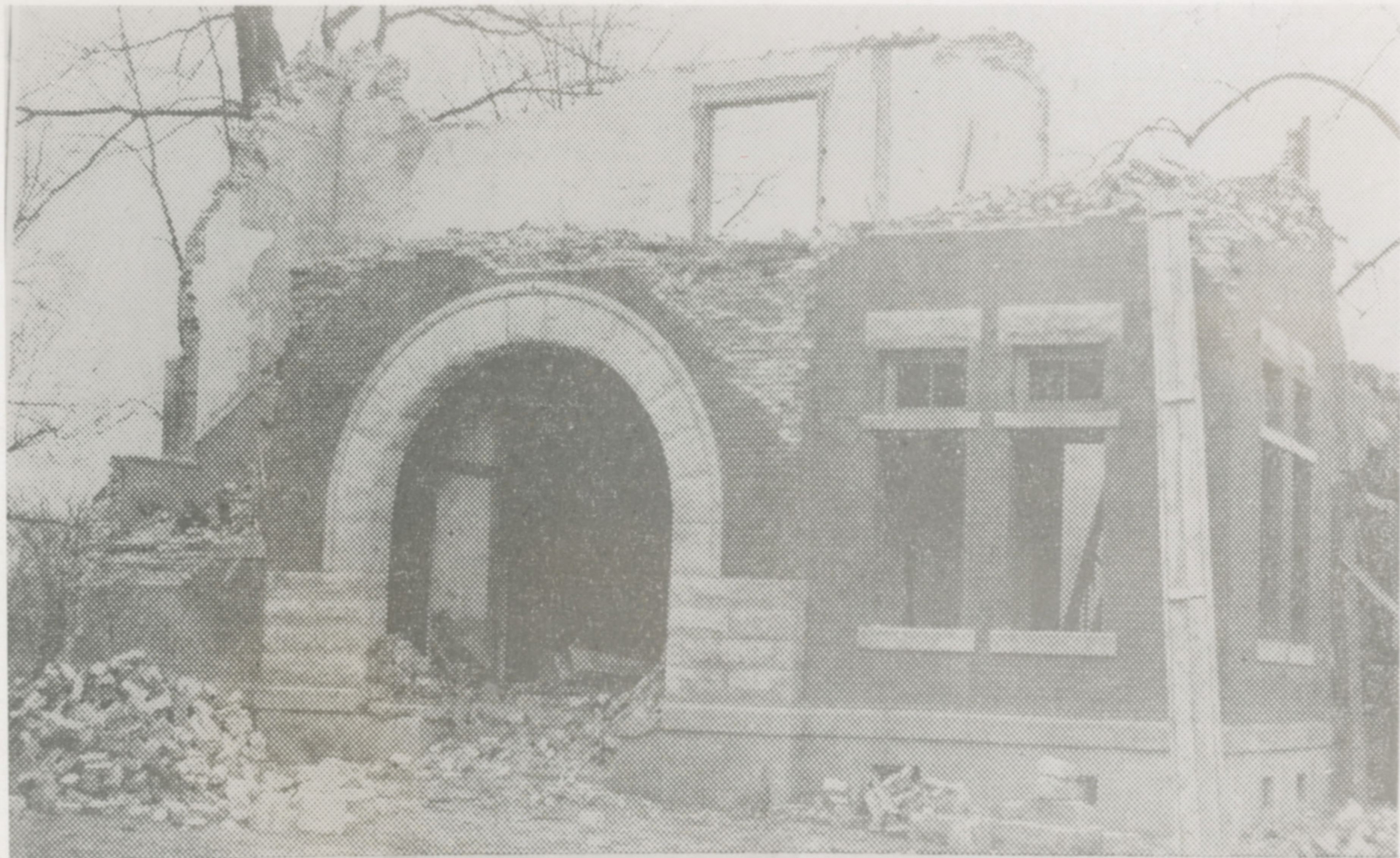
END OF AN ERA —The original courthouse of Coahoma County, Miss., at Friars Point, is being torn down. Clarksdale is now the county seat.
